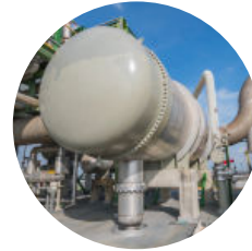
PRESSURE VESSELS AND BOILERS
